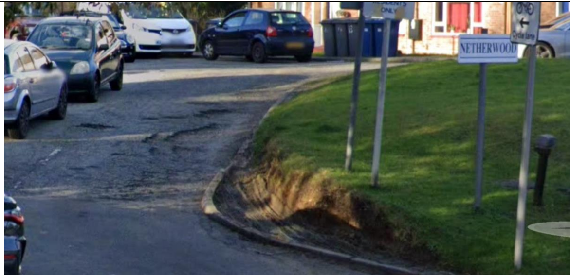
Figure 1 The potholes and state of the road, as well as damage to the side caused by refuse vehicles.
